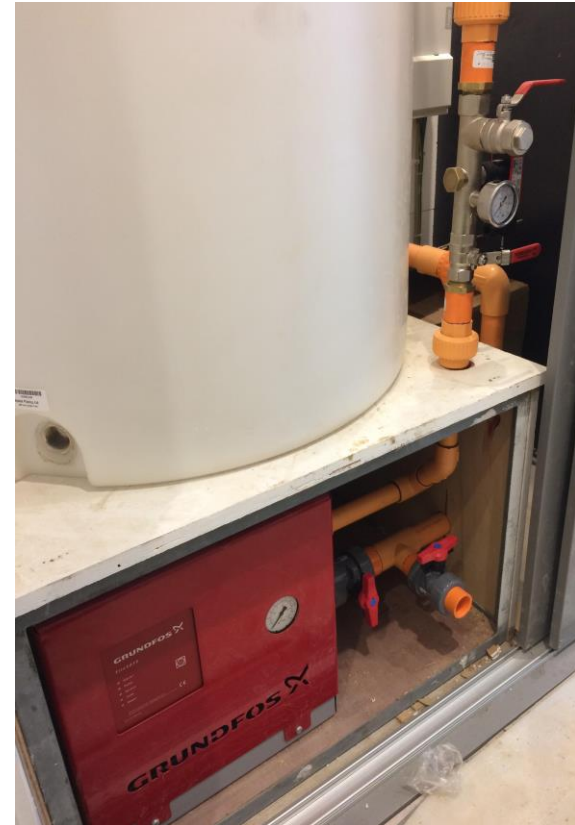
Skid-mounted pump unit with tank over
